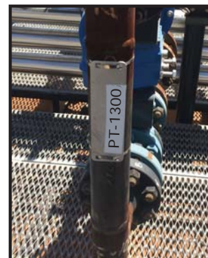
"Flush Mount" Pipe Tag installed at oil field in Bakersfield, Calif.
